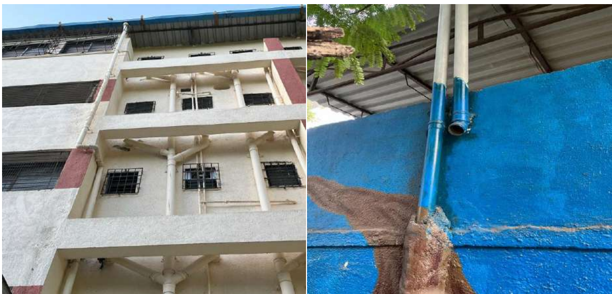
Pipes Originating from Roof Top Discharge Water Down to Ground Area and Garden
