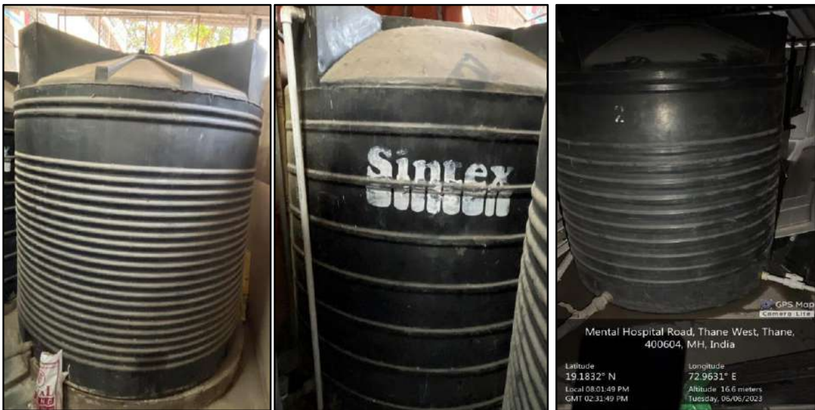
Ground Level Water Tank- 5000 litres each
